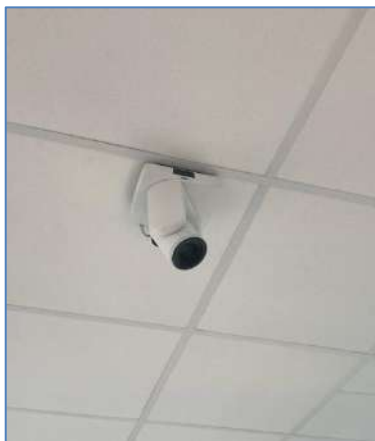
Figure 2 : camera tourelle PTZ.
